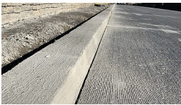
19.11.2024 Grinding of the concrete road surface of the L 2254/B 27 between Kirchheim a. N. and Lauffen a. N.
